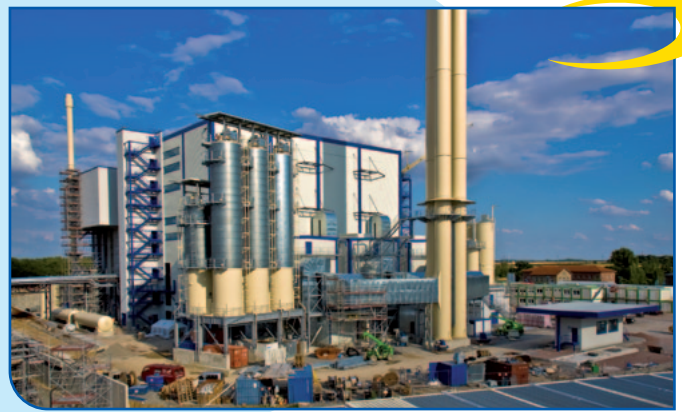
The refuse derived fuel fired thermal power station, which is mainly operated by the Tönsmeier Group, provides process steam.
